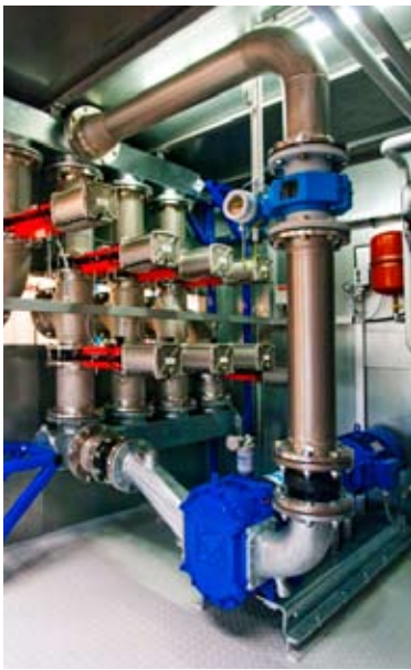
Combined heat and power systems can produce baseload power safely and efficiently
